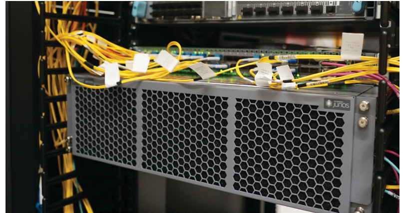
Juniper MX 100003 Router and accompanying QFX5120 ethernet switch located in the Marshfield NOC.
