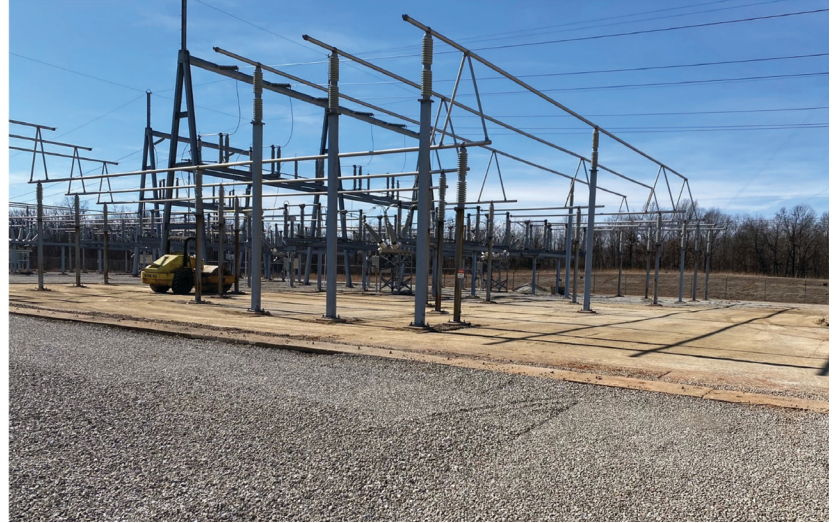
Heavy machinery seen at Ft. Leonard Wood #2 Substation yard compacting the soil in preparation for the layer of gravel to be placed.
