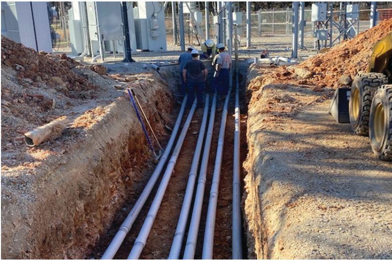
Underground conduit is just part of the infrastructure under a substation which needs to be protected.
