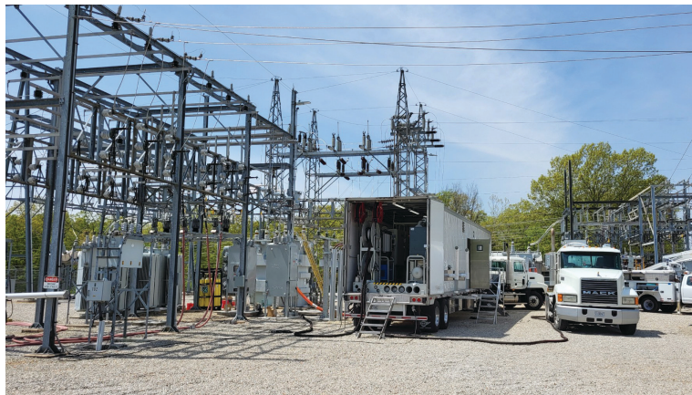
The new oil processing trailer in use at the Gospel Ridge substation.
