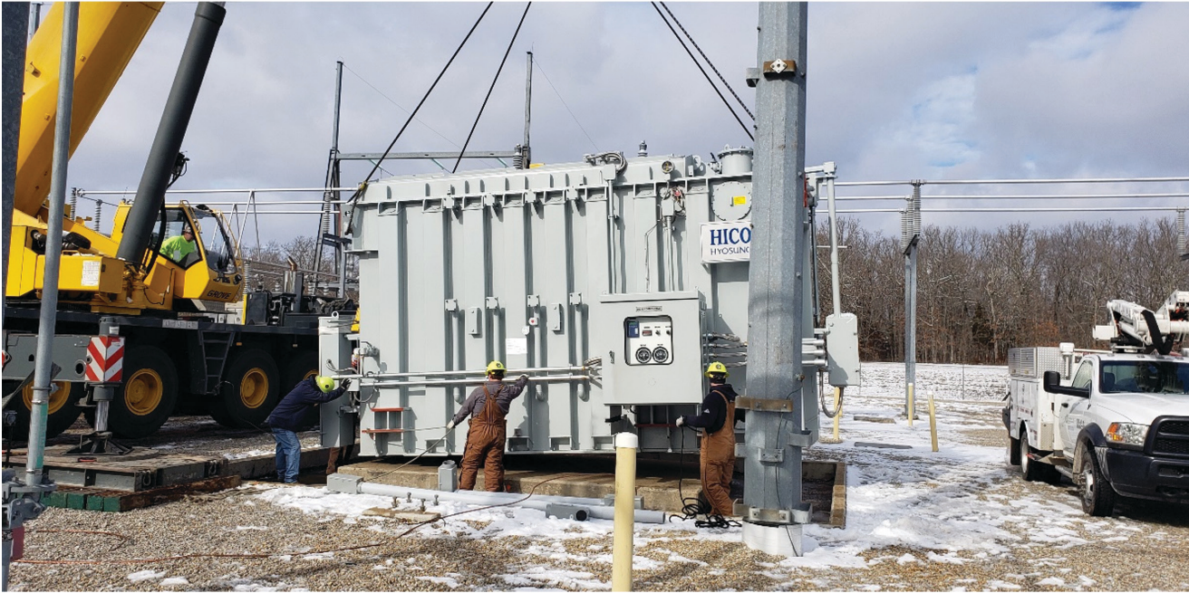
Crane contractors and Sho-Me Substation Mechanics from the Cuba Substation Crew maneuver the reactor onto its final resting place.
